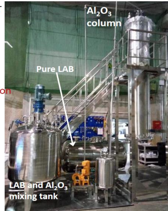
\text{Al}_2\text{O}_3 column pilot plant installed in Daya Bay LS hall
